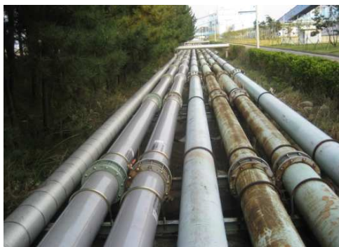
You can see composite pipes on the left and rusted iron pipes on the right side.
